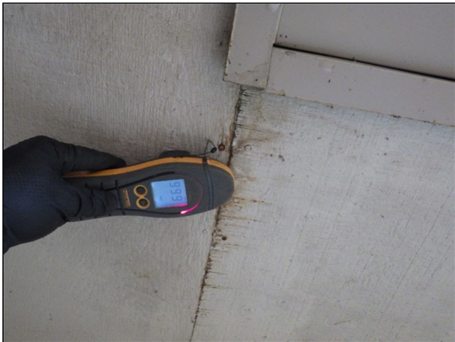
2.5 Item 2(Picture) Moisture meter confirming current leakage.
