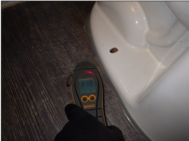
6.0 Item 2(Picture) Moisture meter confirming current leakage.
