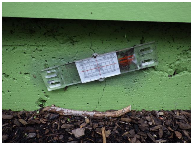
5.2 Item 1(Picture) This is a crack monitor
